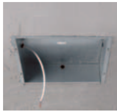
1 pre-installed Downnut conbox
